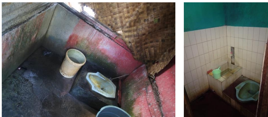
Figure 7. Conditions of the toilet in Mangga Dua Utara District.
