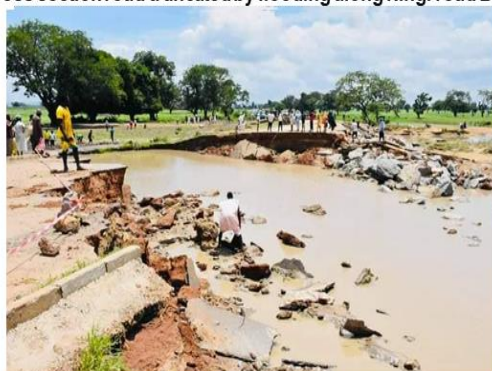
Cross section road truncated by flooding along Ningi road Bauchi.
