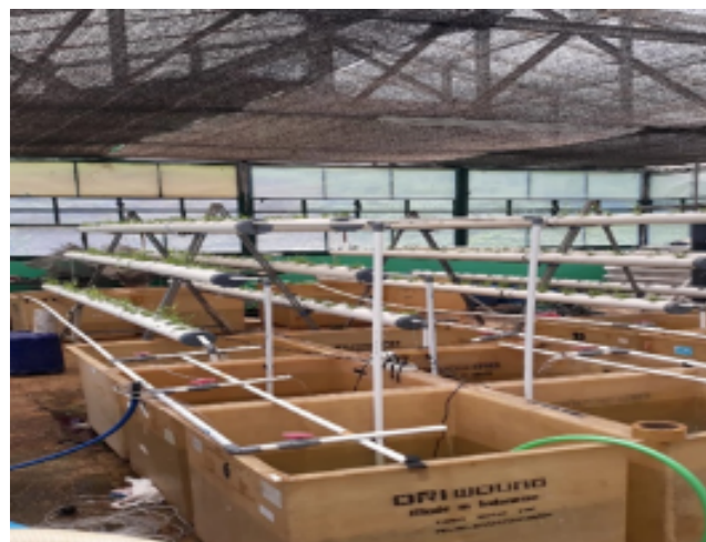
Figure 1. Aquaponic installation used this study
