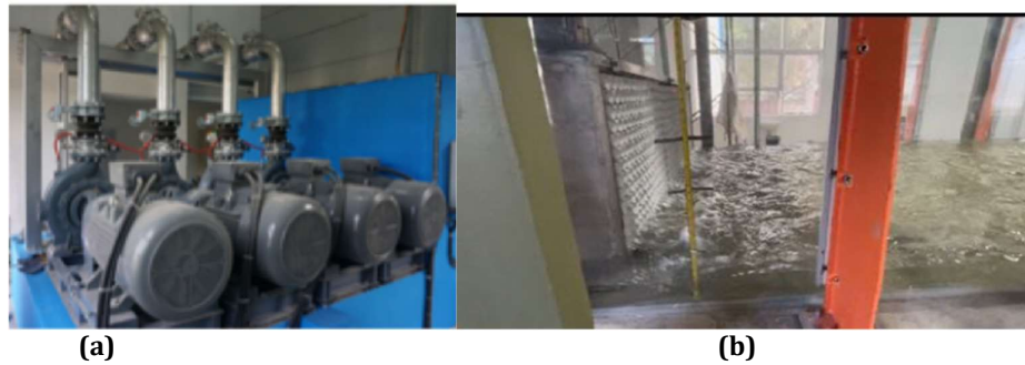
Figure 3. The pump system (a) and the flow straightener (b).
