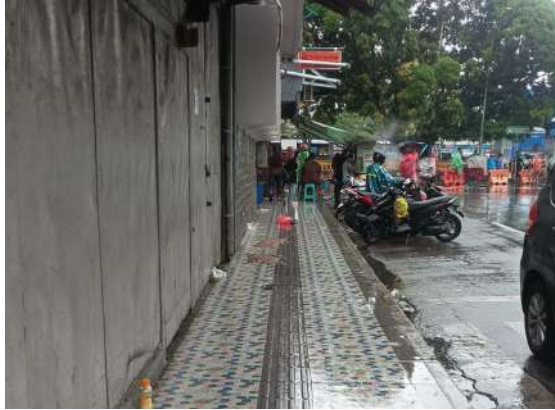
Figure 5. Condition of the Disabled Route in Segment I
