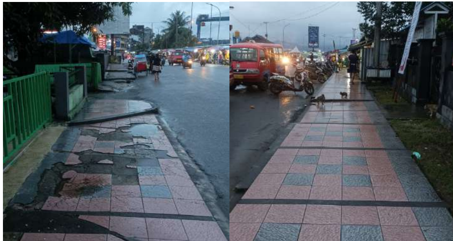
a) Pedestrian Paths in Damaged Condition b) Pedestrian Paths in Good Condition
