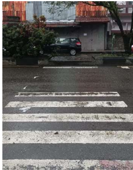
Figure 4. Condition of Crossing Lane in Segment I
